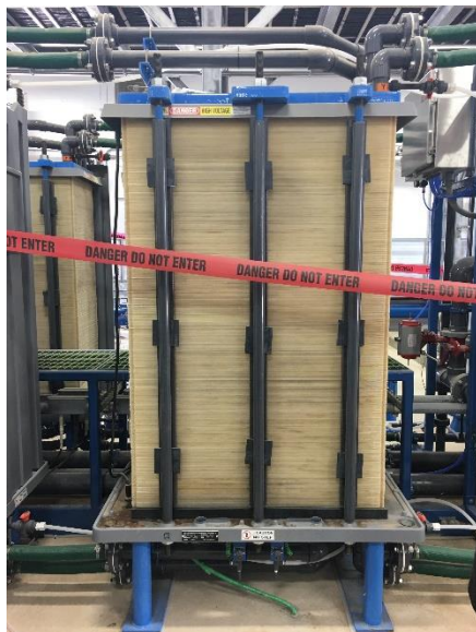
Figure 2: EDR Membrane Filtering
