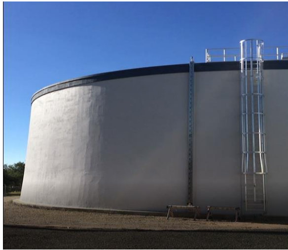
Figure 1: New Groundwater Storage Tank
